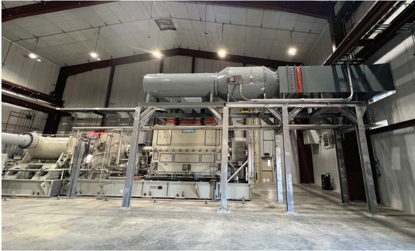
Bi-Con constructed the two-unit electrical driven compressor for the natural gas compressor station project. The unit was built and manufactured offsite, and Bi-Con installed it, connected all the piping and electrical to make it operational. Location is confidential.
