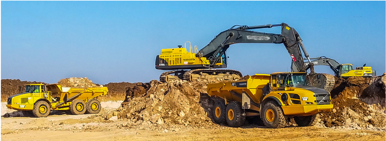
Wondra Construction, a heavy civil contractor involved in wetland restoration, large manufacturing projects and road construction, performs mass grading on a jobsite.
