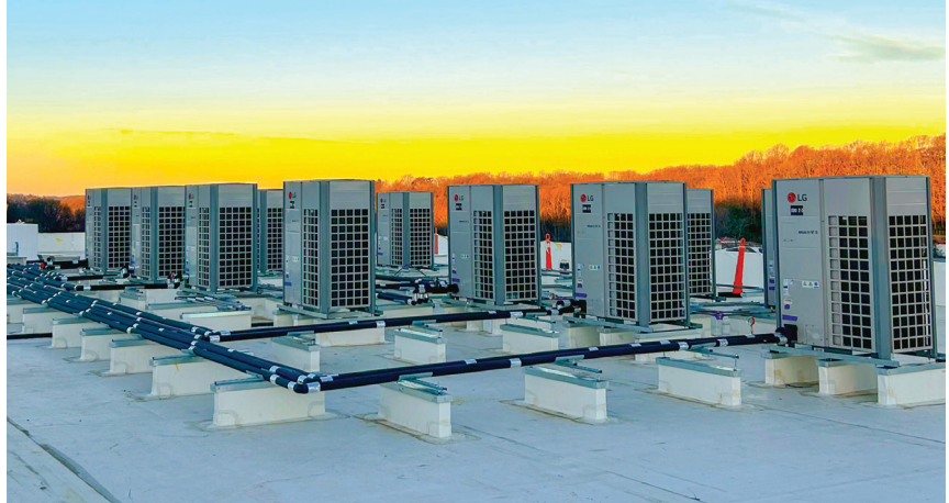
D.J. Wagner Heating & Air Conditioning Inc. was hired as the mechanical contractor on the Northeast Regional Center project in Newtown Square, Pennsylvania, to provide and install an energy recovery unit, two rooftop units, 14 variable refrigerant flow systems with 80 indoor air handlers, and all associated refrigerant piping, condensate piping, ductwork, insulation and controls. This project is anticipated to be completed in the winter of 2026.
